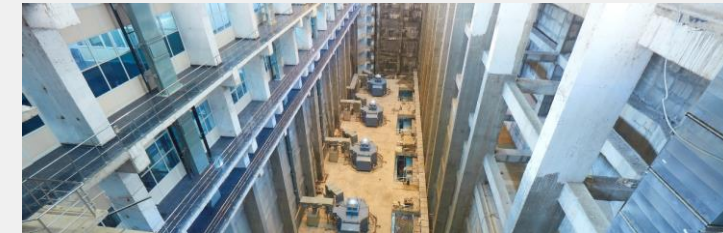
Excitation systems and Motion solutions package for Kaleshwaram lift irrigation project
