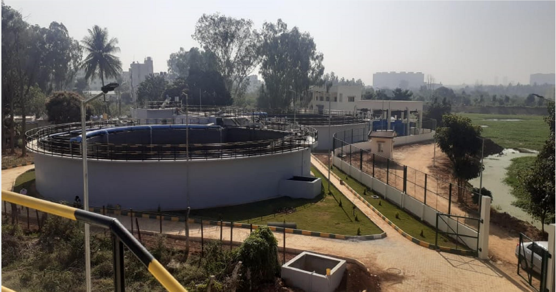
Sewage Treatment Plant established for Rejuvenation of Doddabommasandra Lake at Cost of Rs. 13.5 Crores
