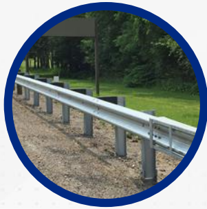
Metal Beam Crash Barrier
