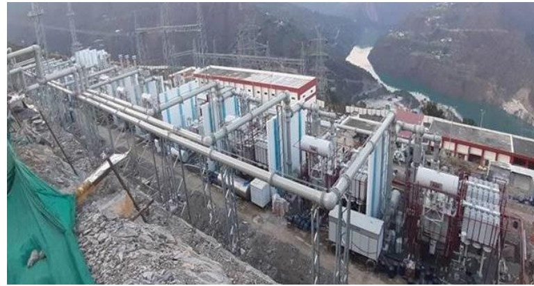
Completed installation of a GIS substation in Uttarakhand, during lockdown
