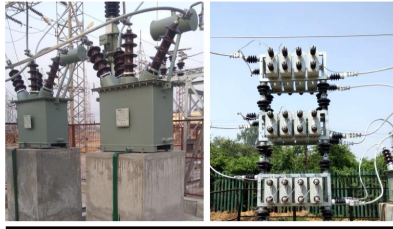
Remote commissioning of capacitor bank in Uttar Pradesh
