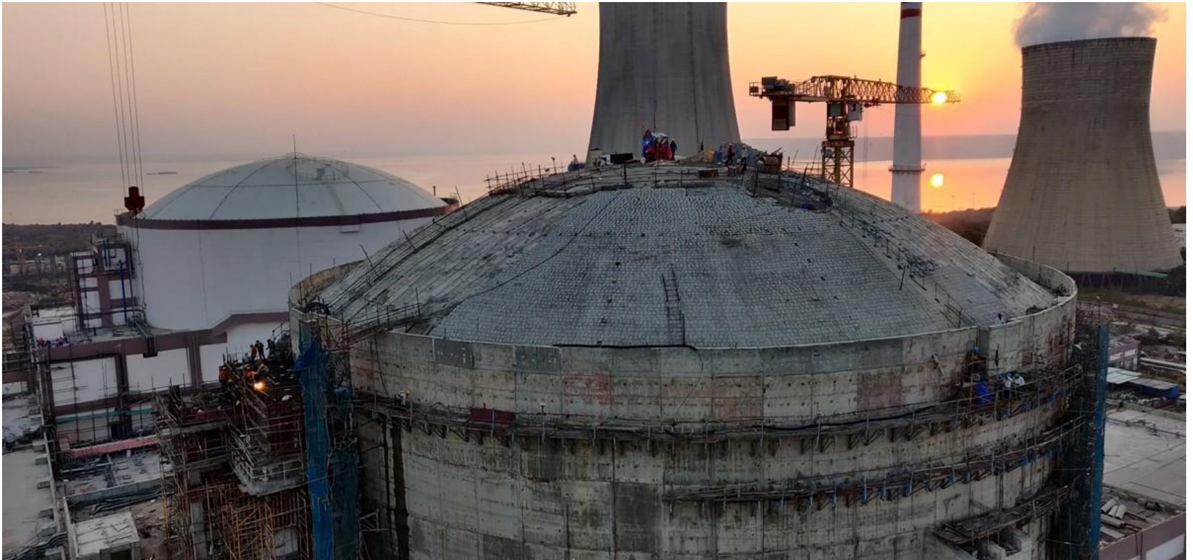
Unit-8 Outer Containment Dome - Aerated tiles work for heat insulation in progress
