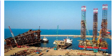
Fabrication Facility, Oman
