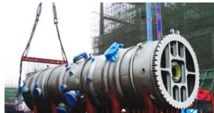
Coal Gasifier for China
