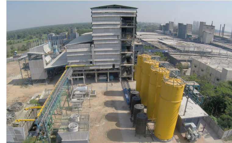
Multiple Effect Evaporator Plant (MEEP)
