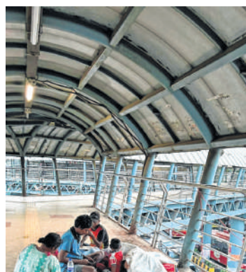
Encroachment on Vikhroli skywalk
