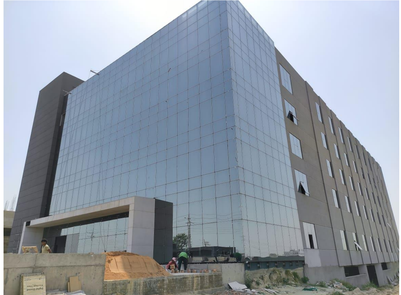
Site Picture: Block I at Plot No 10, Sector 156, Noida, Gautam Budh Nagar, Uttar Pradesh
