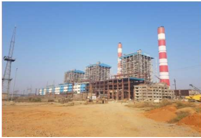
3x660 MW Nabinagar STPP, NPGCL
