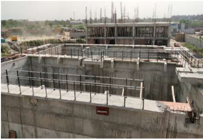
27.5 MLD STP, Networking at Palwal, MCPALWAL
