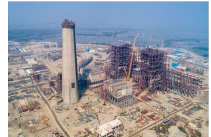
2X660 MW at Rampal, Maitree, Bangladesh-BIFPCL
