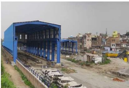
MEMU Shed at Kanpur-RVNL
