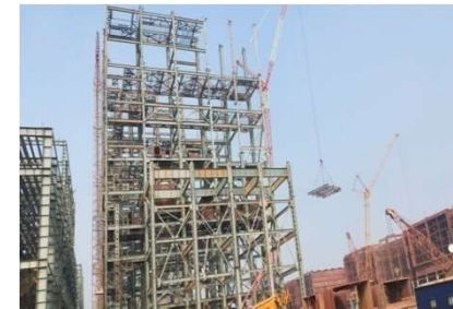
5x800 MW Yadadri TPP, TSGENCO
