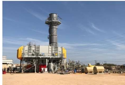
25 MW, Ray Project-RAY International LLC, Oman
