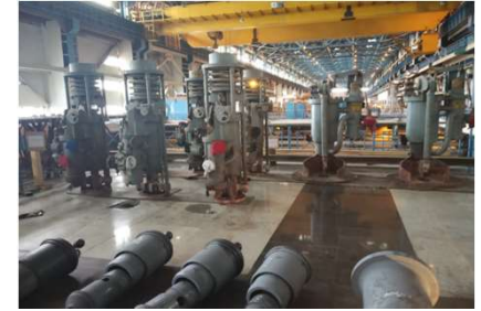
Control & Stop Valves Overhauling Sipat 660 MW
