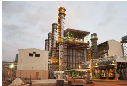
1,390 MW Waad Al Shamal ISCCPP, GE, KSA
