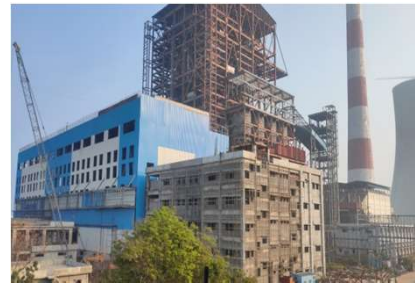
1x800 Mw TPSS, North Chennai, TNGEDCO
