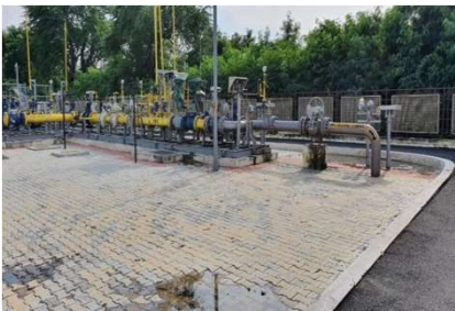
Station Piping at Ennore, IOCL
