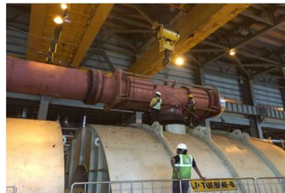
Turbine AOH, 600 MW, Udipi
