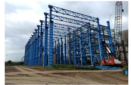
1X660 MW Bhusawal TPS at Maharashtra-MAHAGENCO
