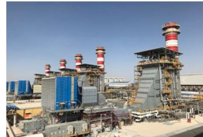
1,519 MW Fadhili CHPP, Doosan, KSA
