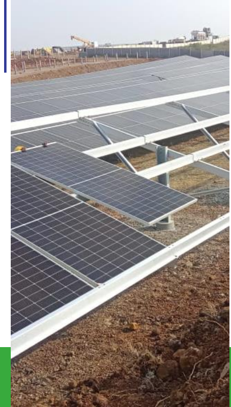
150MWp groundmount project at Ratlam, Madhya Pradesh
