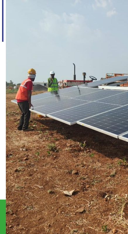
70MWp groundmount project at Jalna
