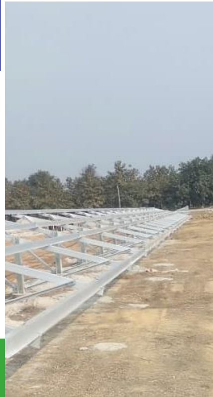
6.5MWp groundmount Project at Raigarh, Chhattisgarh
