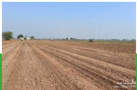
100 MWp at Jamnagar, Gujarat
