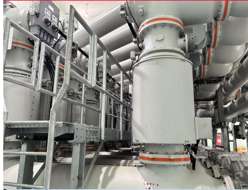
400 kV GIS, 400/220kV 500 MVA ICT, BALCO
