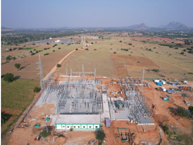
220/33kV AIS Substation for 300MW hybrid generation (solar+wind) at Pavagada
