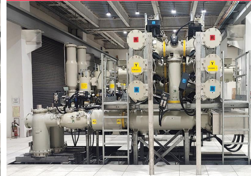
230KV/11kV GIS 2X75MVA Trfo Substation for CTRLS DC, Chennai
