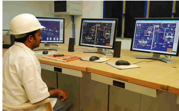
Cement Factory Automation & Control
