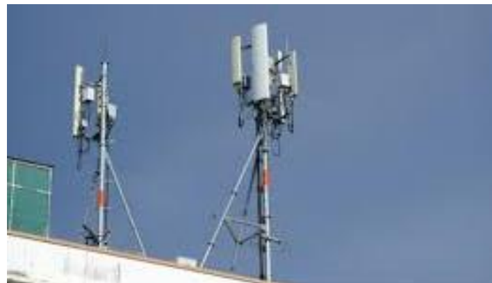
ROOF TOP TOWERS
