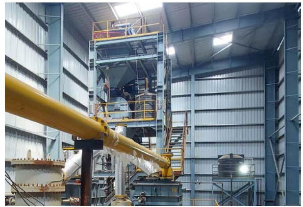
Enhanced Steam Gasification Plant
