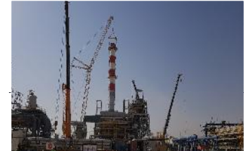
1519 MW FADHILI COMBINED HEAT AND POWER (CHP) PLANT KSA
