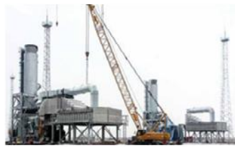
35 MW GT POWER PLANT, KAZAKSTHAN
