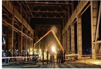
1X800 MW TPSS, CIVIL, STRUCTURAL AND ARCHITECTURAL WORK STAGE-3, NORTH CHENNAI, BHEL
