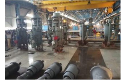
CONTROL & STOP VALVES OVERHAULING SIPAT 660MW
