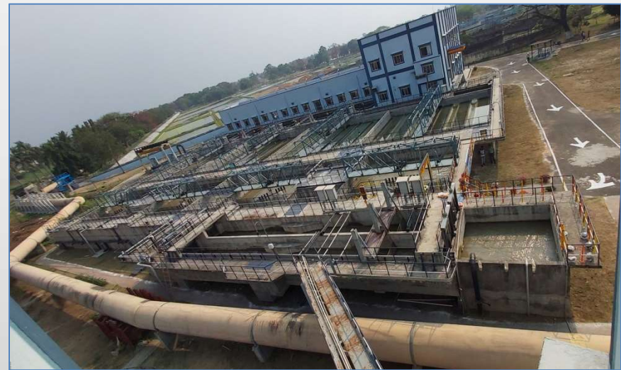
Palta WTP, West Bengal
