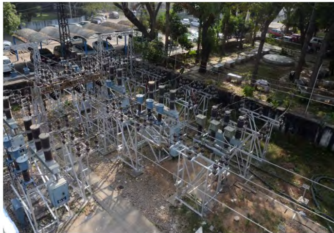
33kV GSS after Maintenance
