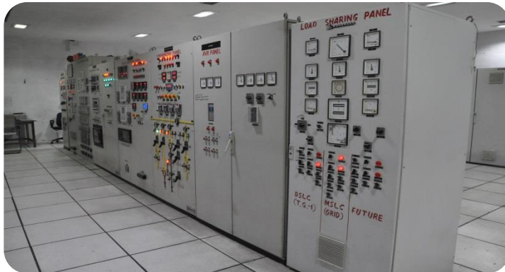
Cogeneration Control Panel
