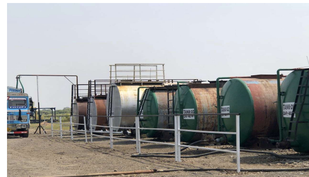
Jyoti I – Oil Storage
