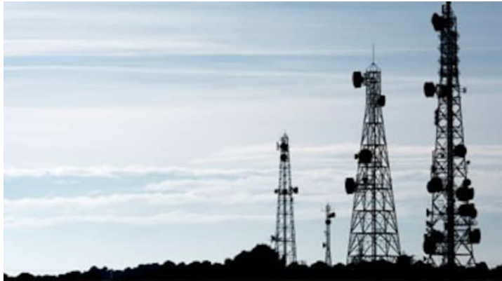
GROUND BASED TOWER
