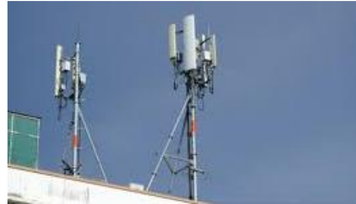
ROOF TOP TOWER
