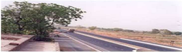
Project: Four laning of NSEW corridor of Agra Dholpur section of NH-3
