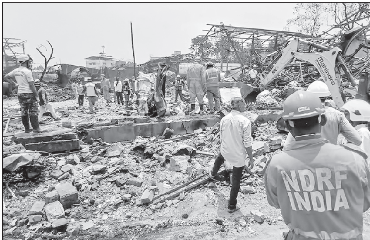
NDRF personnel at the site where a boiler exploded at the chemical factory on Thursday, in Thane on Friday.
