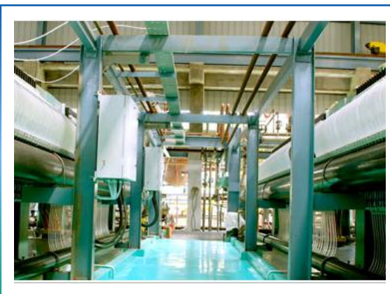
Caustic Soda manufacturing, Karaikal, Puducherry
