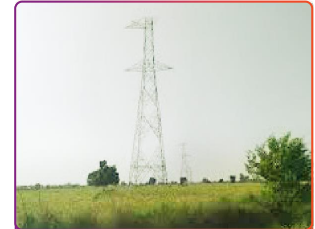
765kV Ghatampur TPS-Agra SC line
