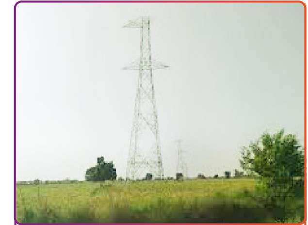
765kV Ghatampur TPS-Agra SC line
