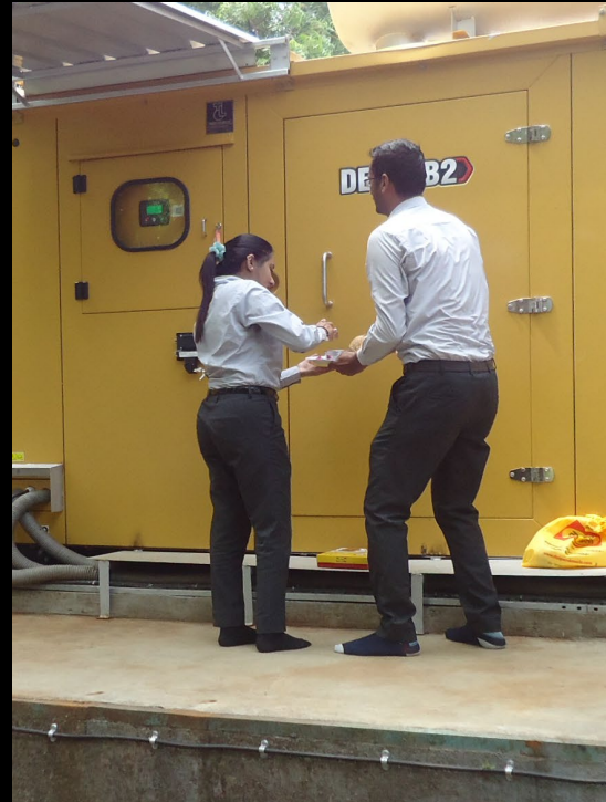
Newly Installed Power Back Up Facility
