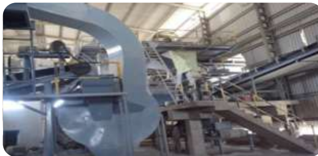
Unit 2– Granulation Plant
