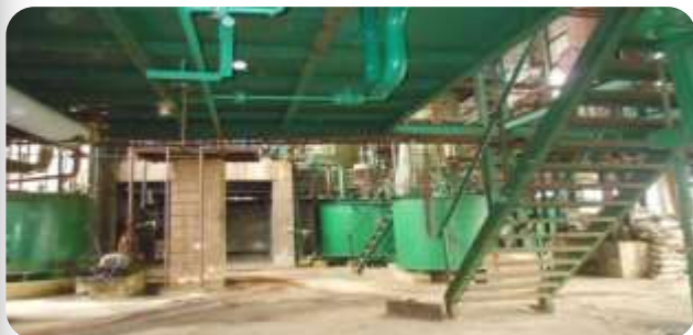
Sulphuric Acid Plant
