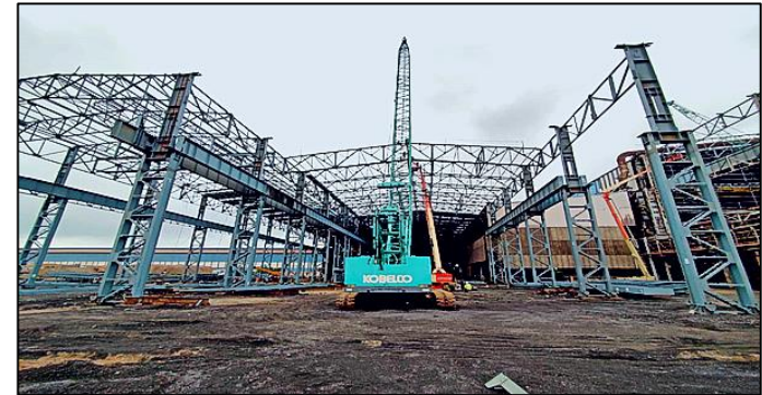
SMS-2 at JSW BPSL
