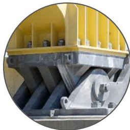
Bearing & Expansion Joint
