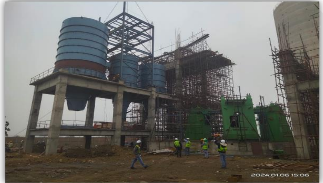
Hopper & Cement Mill
