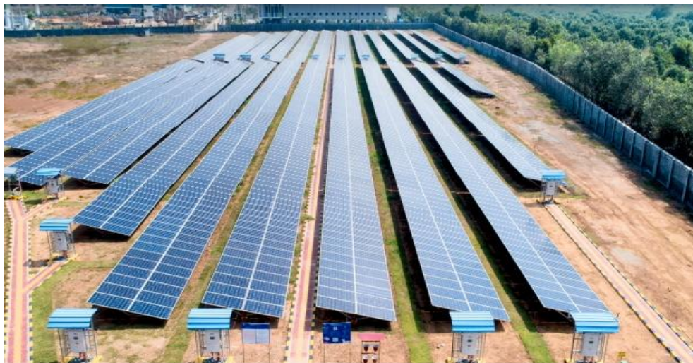
Solar & Wind Installations across plants
