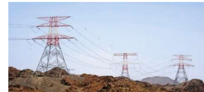
Transmission Lines, Fujirah, Dhaid
