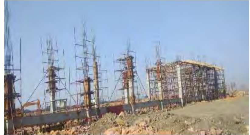
Engine line building
