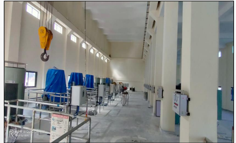
Pumping Station at Bhama Askhed, Pune
