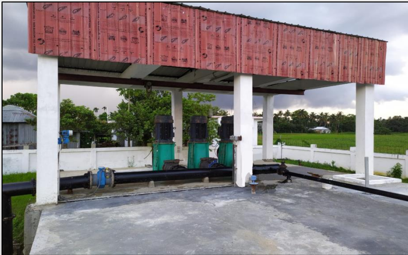
Clear Water Pumps at Rampur, Agartala
