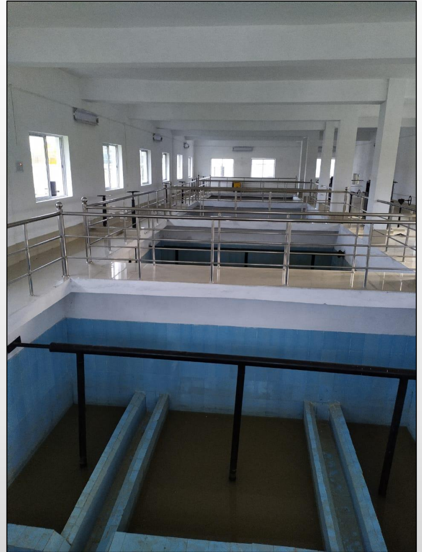
Filtration Plant at Rampur, Agartala
