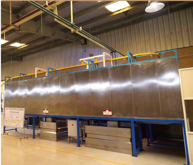
Gas Fired Baking Oven
