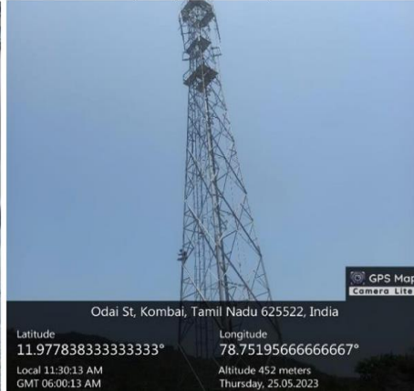
4. Tower AT (Acceptance Test)
