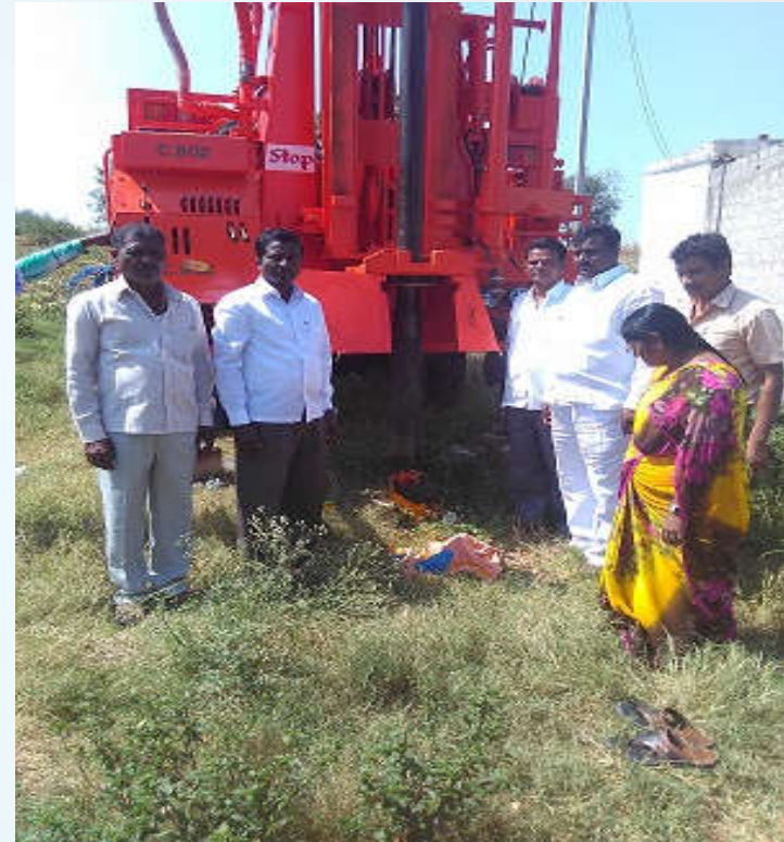
Construction of borewells, storage tanks, water distribution pipelines and RO drinking water plant at Chowdammagutta Thanda village in Mehaboobnagar district, Telangana by Hyderabad Unit
