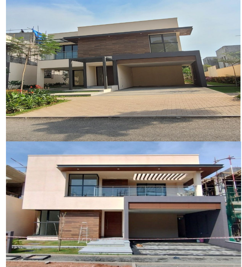
Villa completed in Q4 is 3 Nos and total completed villas are 6 Nos Total SBA completed in Q4-FY23 – 9,630 sft
