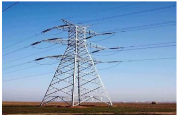
Power Transmission Tower
