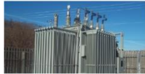
Transformer & Sp Oil
