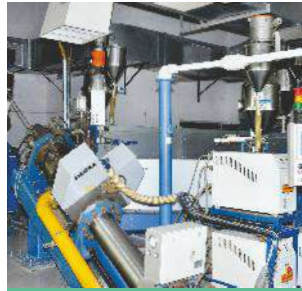
550 kV Maillefer HVCV Insulate Line
