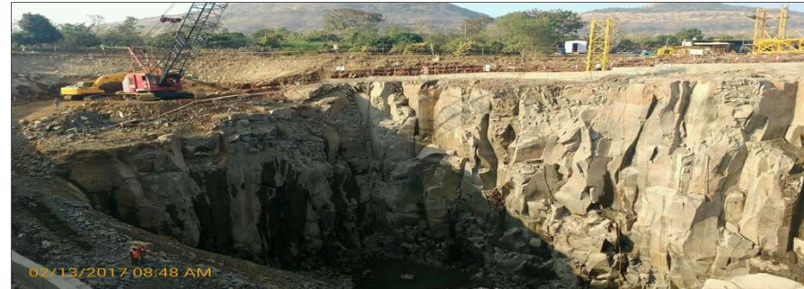
Bhama Askhed Water Supply Project
