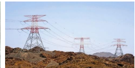
Transmission Lines, Fujirah, Dhaid
