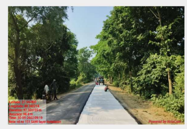
Laying of Paving fabric and Providing BC / PQC over the stabilized Layer
