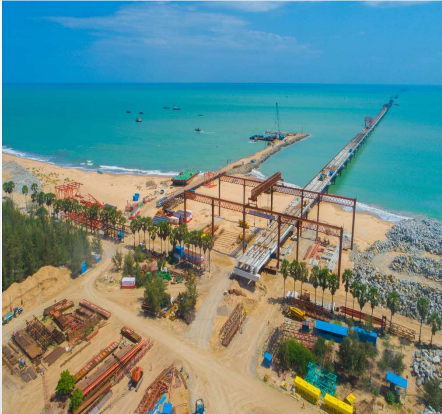
Udangudi, Tamilnadu Power Project
