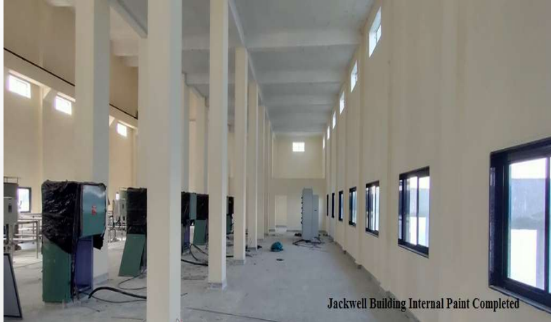
Bhama Askhed Water Supply Project
