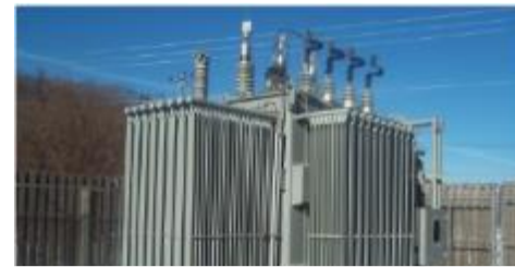
Transformer & Sp Oil
