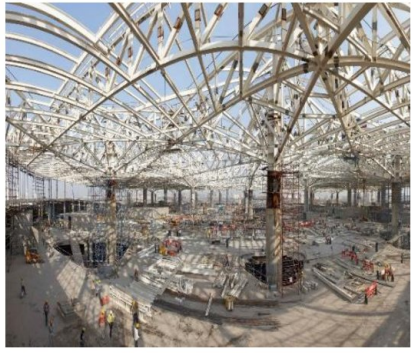
Curtain Walling Structure at Mumbai Int'l Airport
