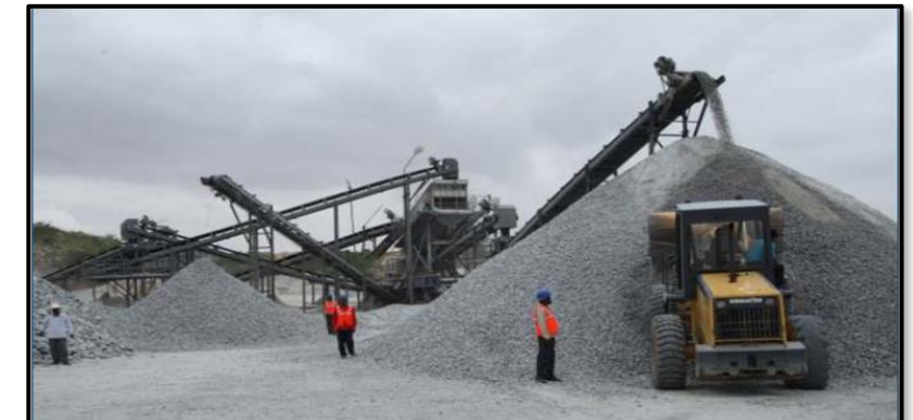
250 TPH Nawa Crushing Plant
