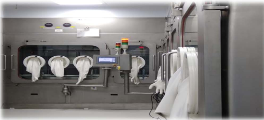
Filling facility - Fully Automated
